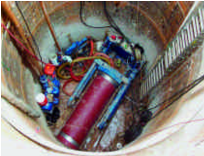
Mission Clay No-Dig pipe in 8-ft lengths was installed along the majority of the alignment.
