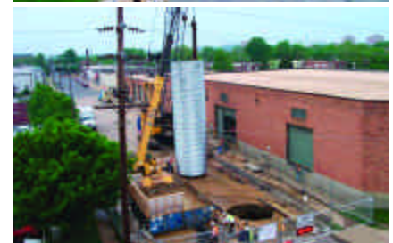
To avoid dewatering and thus reducing risk of settlement and consequent damage to nearby utilities, roadways and buildings, Shirley Contracting utilized a drilled slurry method (subcontracted to Case Foundation Co.).
